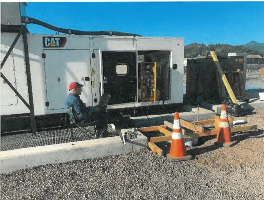
Generator technician monitoring power delivery and communications (6/19/19)
