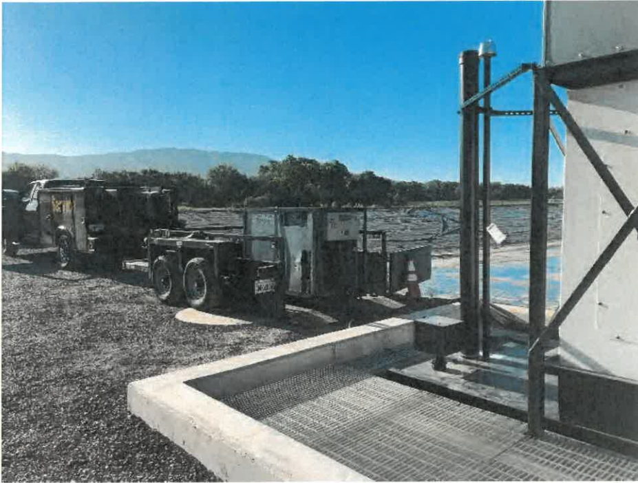
Load bank used to test standby generator (6/19/19)
