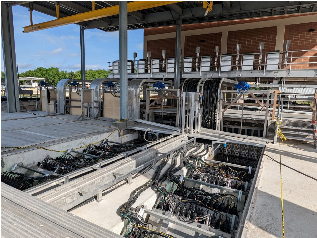
Figure 17 Trojan UVSigna 2-Row System (JEA, Florida)
