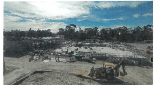
Miramar Clearwells Chlorine Contact Chamber
